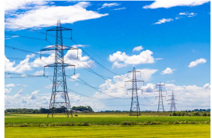
Pylons carry overhead power cables
